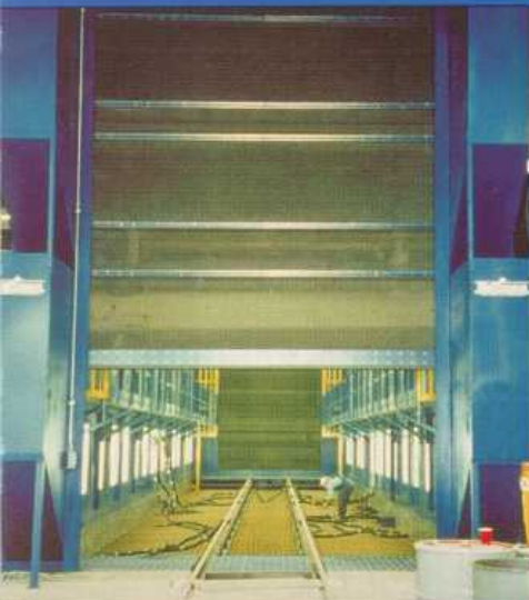
Full Reclaim Blast Room with Recessed Floor, Powered Rubber Roll-up Door and Man Walkways
